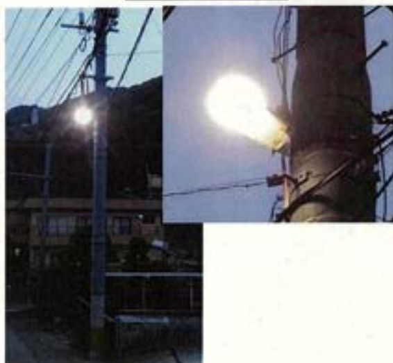
LED 街路灯 (電柱共架)
